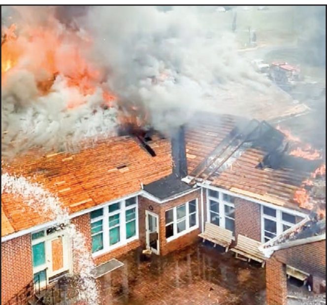
The Dining Hall demolition project at Young Harris College offered invaluable training opportunities for area firefighters last month. Photo/Submitted
